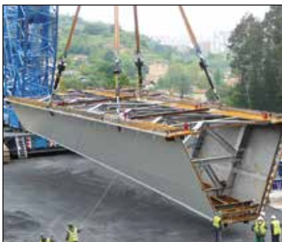
▼ Bridge segments are hoisted from the ground, being positioned with a 4-point SyncHoist system with fully monitored cylinders.
