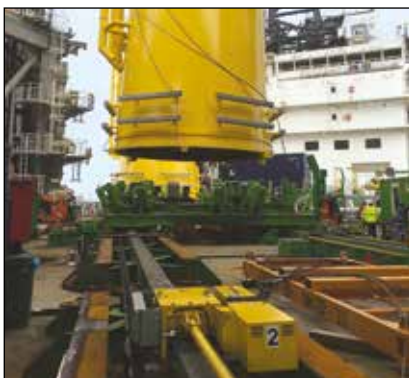
▼ The trolley system speeds up offshore wind transition piece load out: the transition pieces are positioned in the clamping frames and moved along the track.
