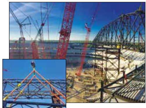
▼ Enerpac SyncHoist system in use during roof truss picks: precise lift and positioning of stadium retractable roof trusses. 33 trusses weighing between 450 - 750 ton.
