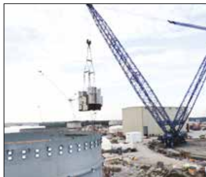
▼ Rigging engineers used the SyncHoist system to precisely monitor and adjust each lifting point independently, or together in a synchronized manner to position the 1140 ton nuclear plant module.
