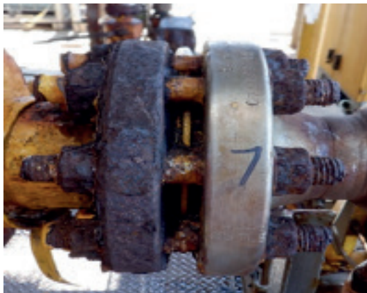
Fig. 1: Galvanic Corrosion Effect on Joint Components with incompatible materials requiring Hot Bolting to upgrade bolts
